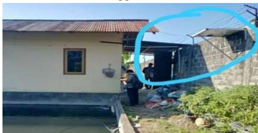
Gambar 3. Panel Surya terpasang
